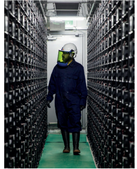
Broxburn Energy Storage System
